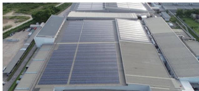
Mega solar panels installed at TRT (Thailand)
