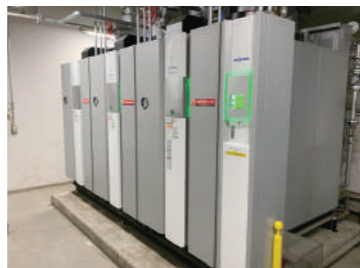
■ Boiler for heat source of air conditioning
