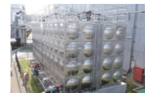
Batch type final effluent tank
